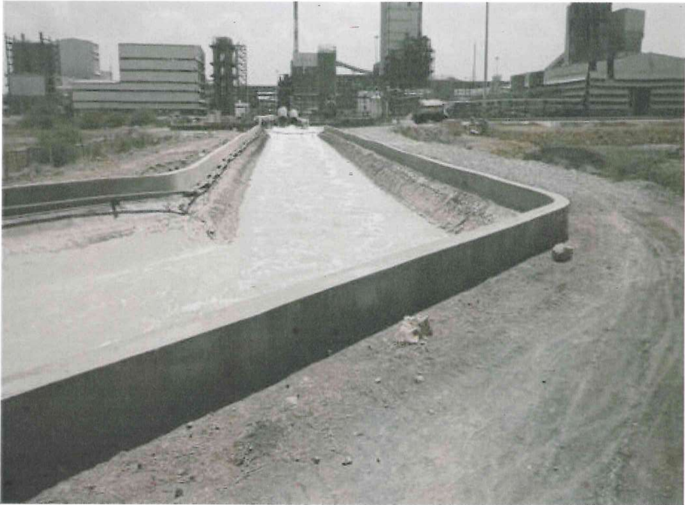
Construction of Parapet wall (1.5 feet height) covering mixing pond and channel length between mixing pond and outfall discharge chambers
